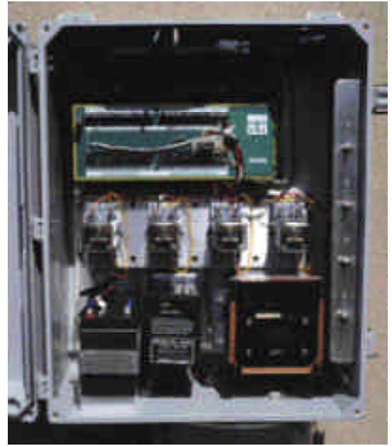
Event-Actuated, Early-Warning Alarm System Monitoring Industrial Effluent. The 6200 Monitors and Controls Pumps Based on pH and Dissolved Oxygen
