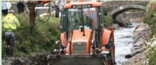
Flooding at Boscastle P1-2
